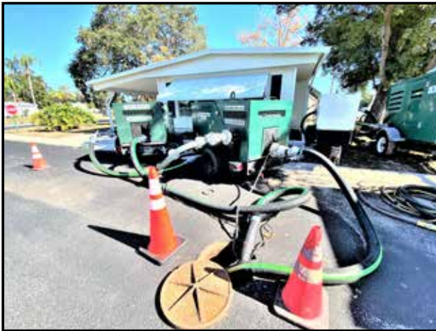
Bypass pumps were used during Lift Station Rehab on Royal Palm in December 2020
