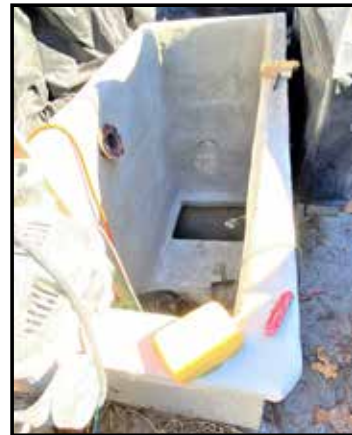
Lift Station Re-lining. This rehab project was to fix problems with overflow that occurred during periods of heavy rains.
